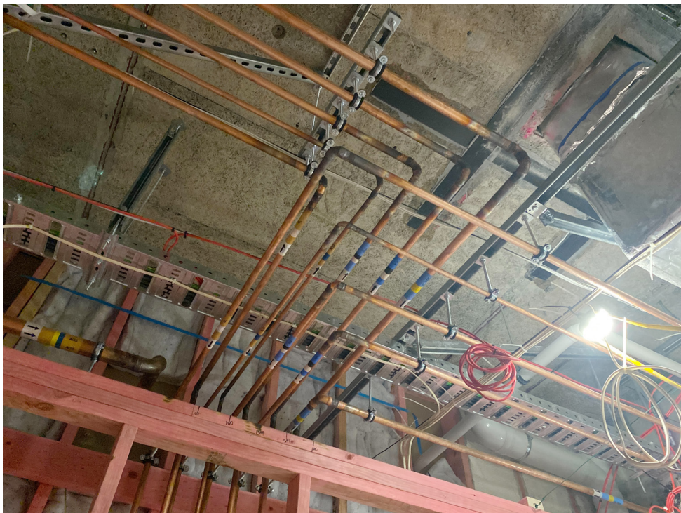
SPIRE ceiling ducting for heating, medical gases, energy and water.
